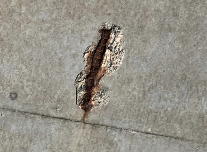
Figur 16. Tunnel N, detalj korrosion, armering.
